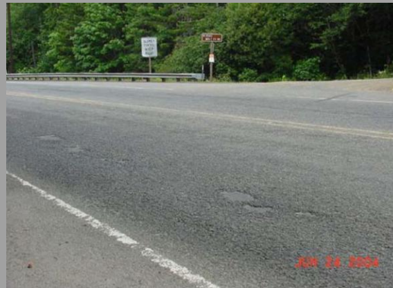
Oxidation and Raveling – High
