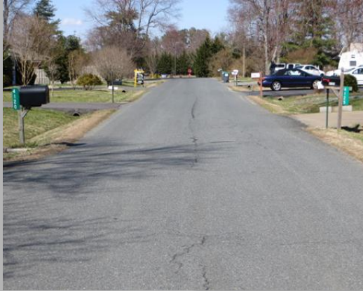
Fatigue Cracking - Low
