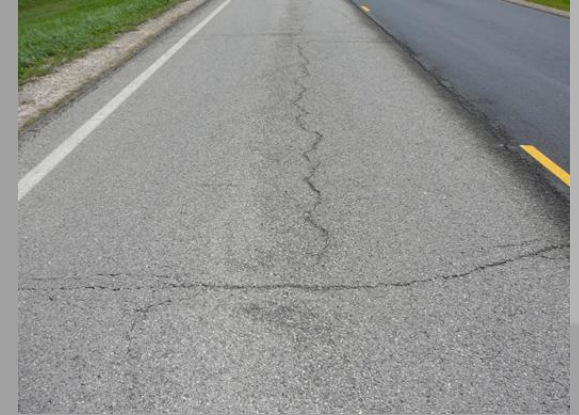
Longitudinal & Transverse Cracking - Low
