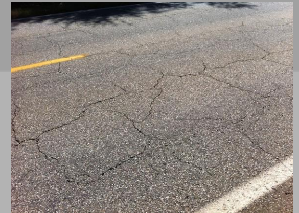
Longitudinal & Transverse Cracking
