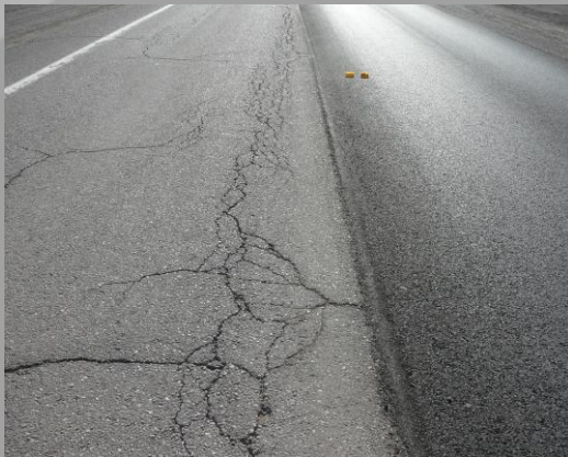
Fatigue, Longitudinal & Transverse Cracking
