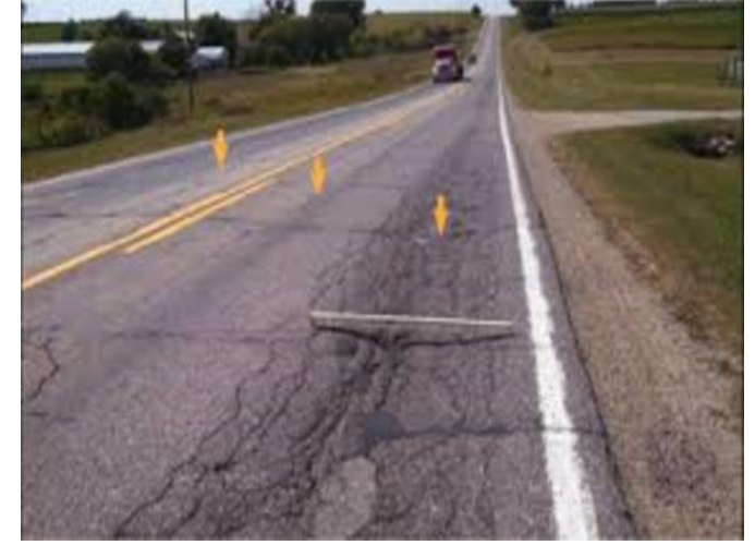
Fatigue Cracking with Rutting – High With High Traffic Volume
