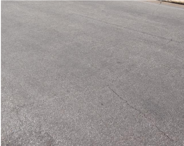
Fatigue Cracking - Low
