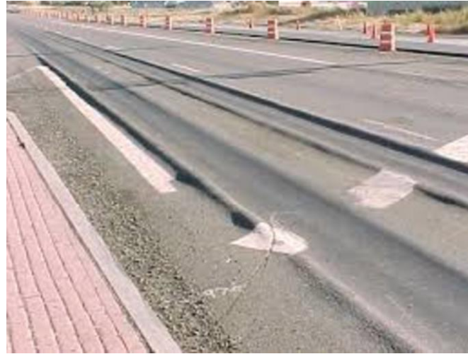
Rutting – High With High Traffic Volume
