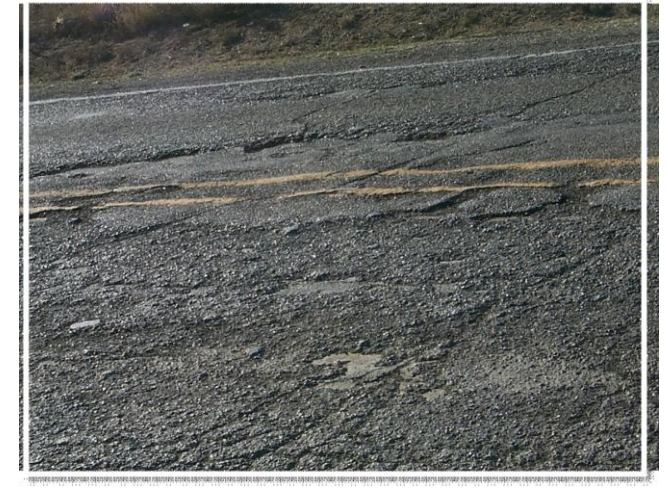
Oxidation and Raveling - High
