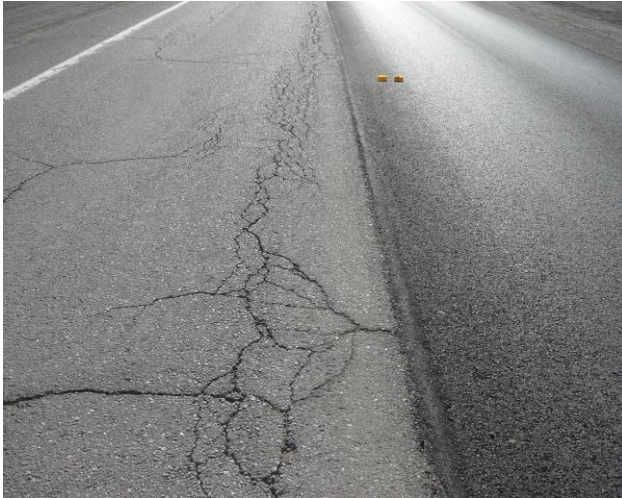
Fatigue, Longitudinal & Transverse Cracking – Moderate
