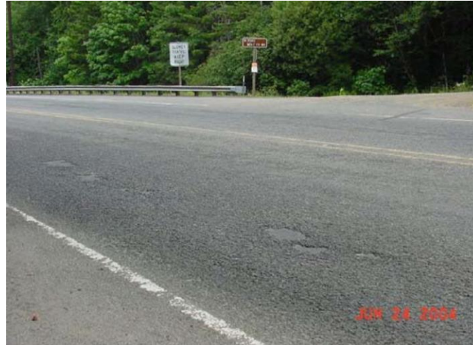
Oxidation and Raveling – High
