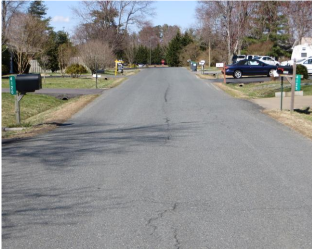
Fatigue Cracking - Low
