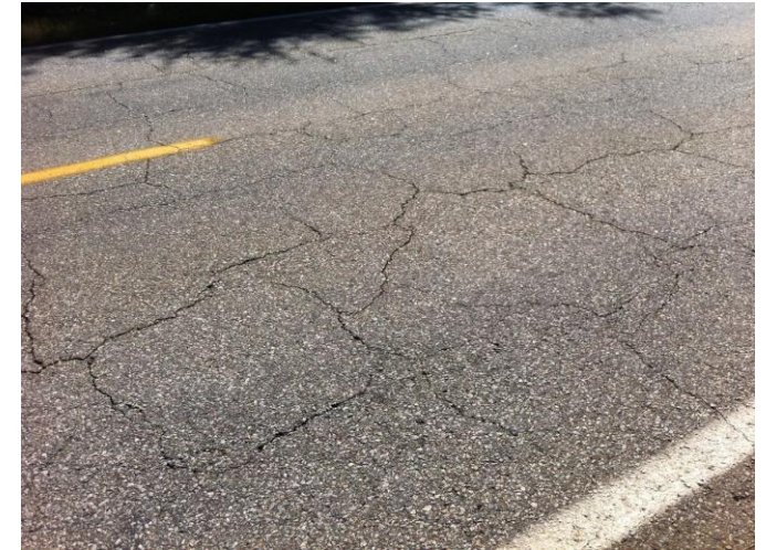
Longitudinal & Transverse Cracking Moderate
