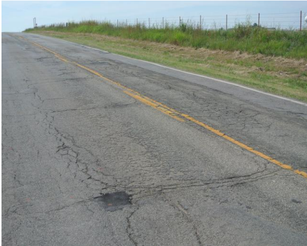
Fatigue Cracking – High Potholes
