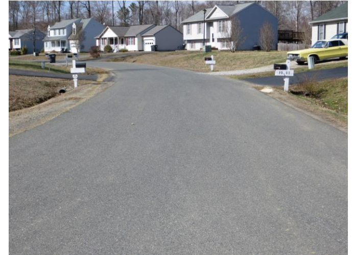
Preventive Maintenance Candidate
