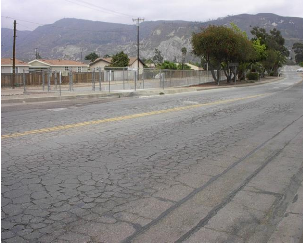
Fatigue Cracking – High With High Traffic Volume
