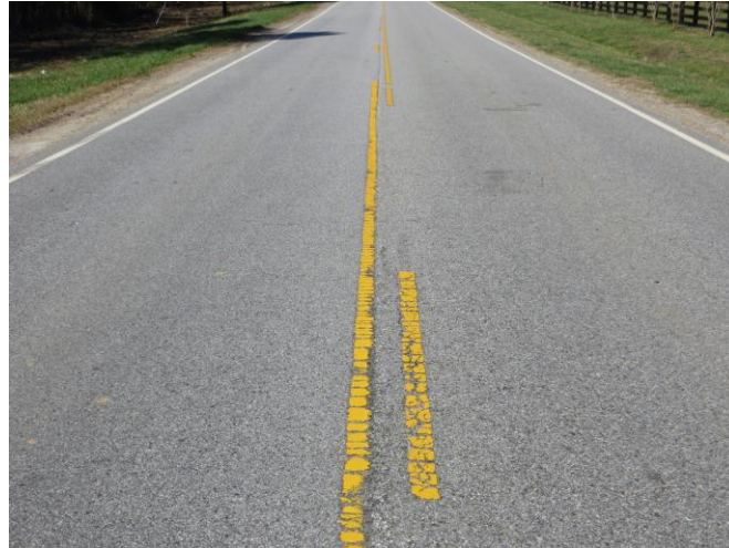
Oxidation and Raveling – Low
